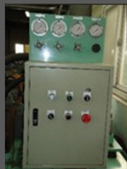
Breaker Final Test
